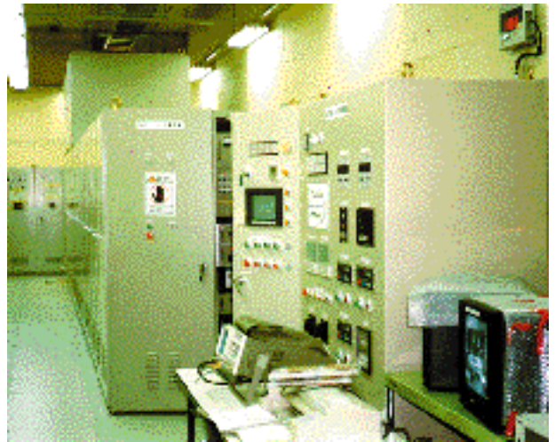
Fig. 2 The modulator installed in the electron beam sterilization facility.
