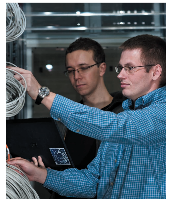
Milosz Hulbój (left) and Ryszard Jurga (right) working on the network switches in the CERN Computer Centre
