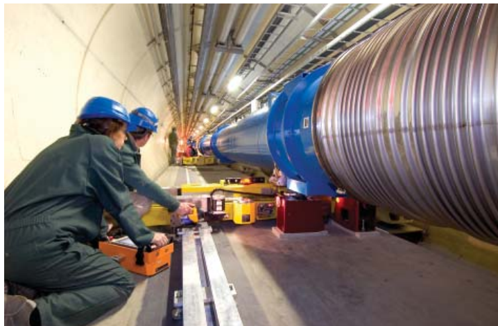
Installation of the first LHC dipole magnets in March 2005
